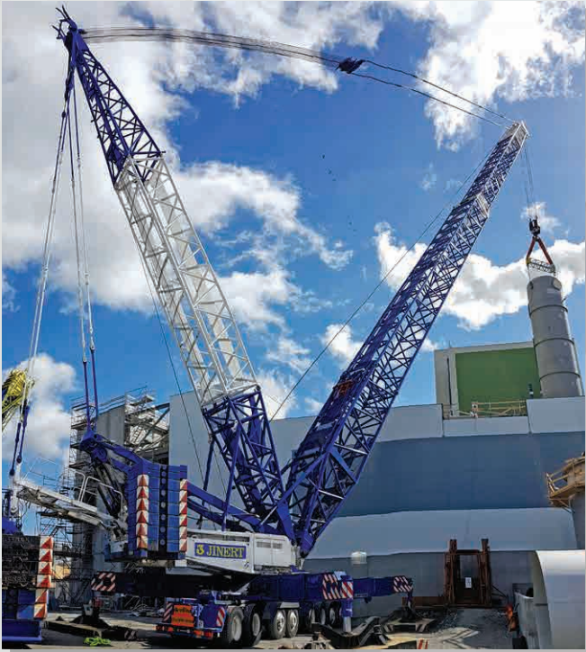
Erection of evaporation plant at paper mill owned by Södra Cell Mörrum, Sweden
