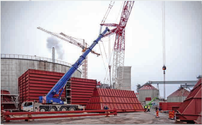
Supply, erection and thermal insulation of the gas treatment plant in Västerås, Sweden
