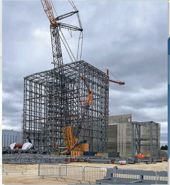
Waste incineration plant in Ferrybridge, UK
