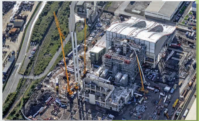
Waste incineration plant owned by Trident Park in Cardiff, UK
