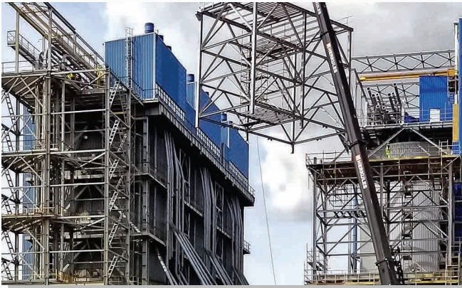
Erection of flyovers and slag transport system in Opole Power Plant, Poland
