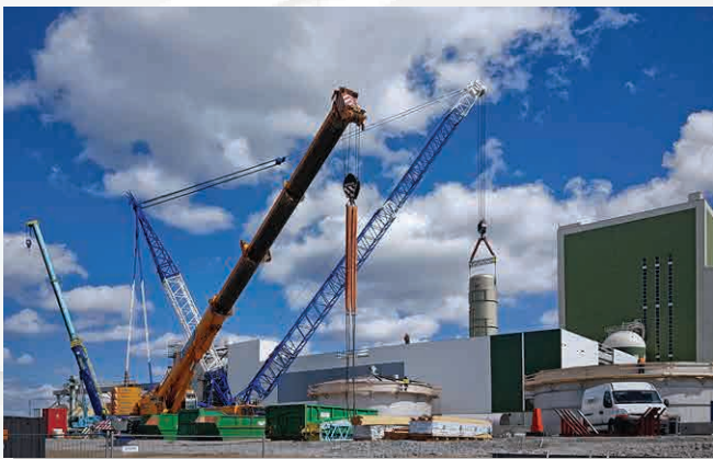
Erection of evaporation plant at paper mill owned by Södra Cell Mörrum, Sweden
