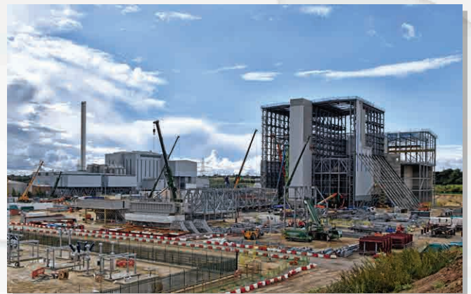
Waste incineration plant in Ferrybridge, UK
