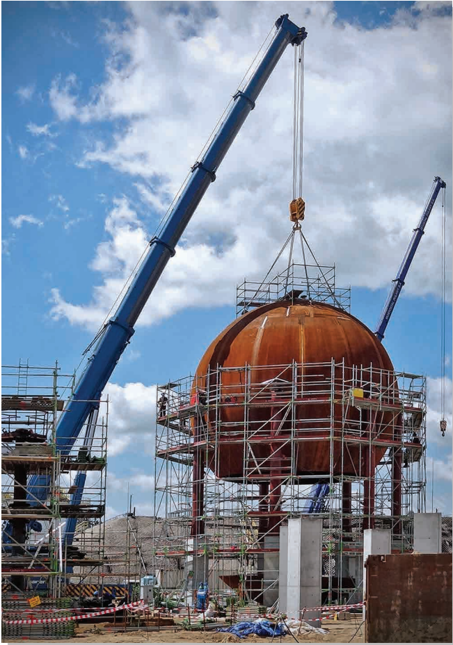
Spherical tanks Orlen in Plock, Poland
