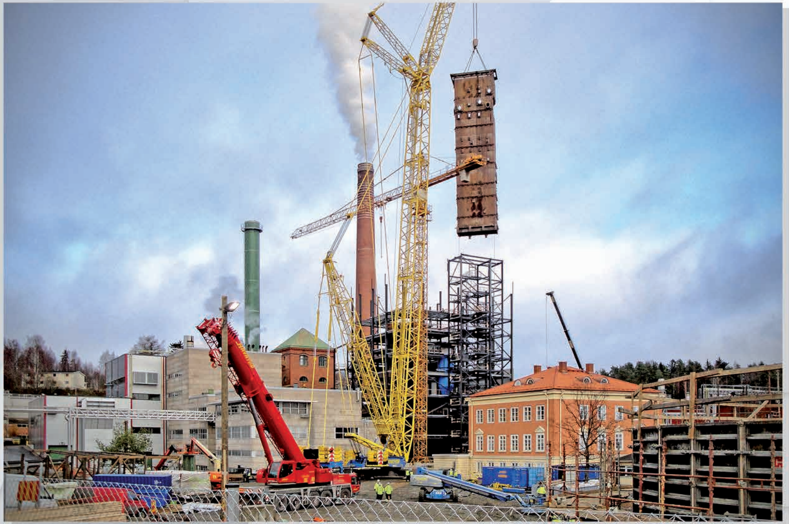
Erection of biomass BFB boiler together with equipment and low-pressure pipelines at CHP plant owned by HaVo in Kyröskoski, Finland
