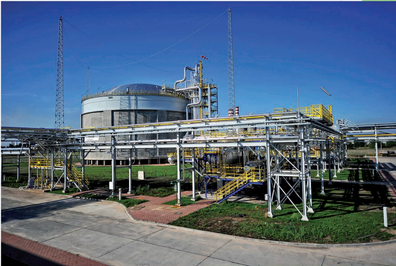
Steel structure delivery and erection as well as installation of equipment and technological piping for the project: Urea and ammonium sulphate based solid fertiliser production at Zakłady Azotowe "Puławy" S.A., Poland
