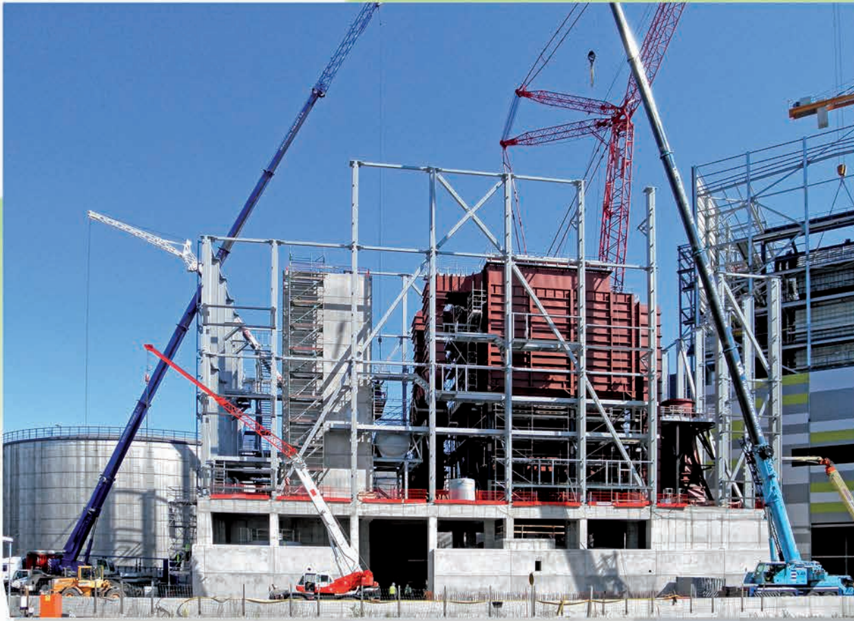
Supply, erection and thermal insulation of flue gas treatment plant in Västerås, Sweden
