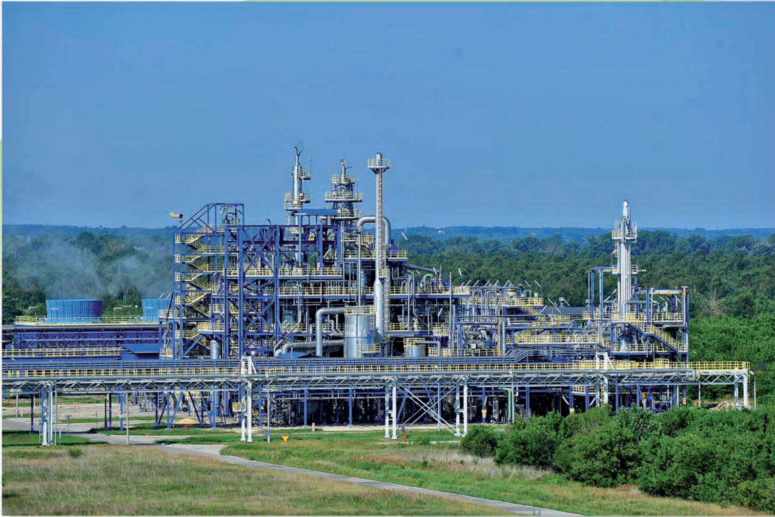
Construction of Melamine Manufacturing Plant II at Zakłady Azotowe "Puławy" S.A., Poland – project executed as General Contractor
