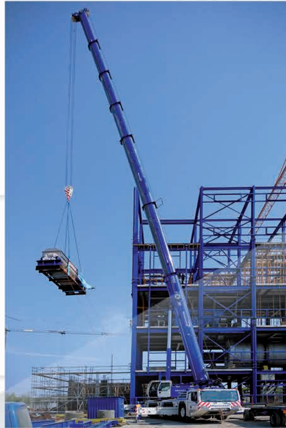
Steel structure delivery and erection as well as installation of equipment and technological piping for the project: Ammonium nitrate based granular fertiliser production plant at Zakłady Azotowe "Puławy" S.A., Poland
