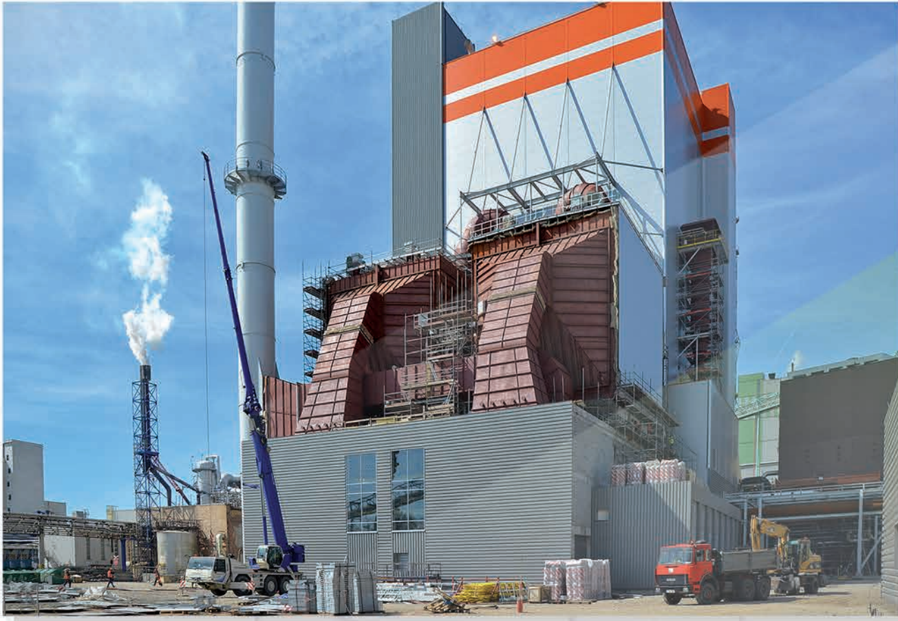
Erection of soda recovery boiler (2 300 tds/d) and two ESPs at paper mill owned by Mondi Świecie, Poland
