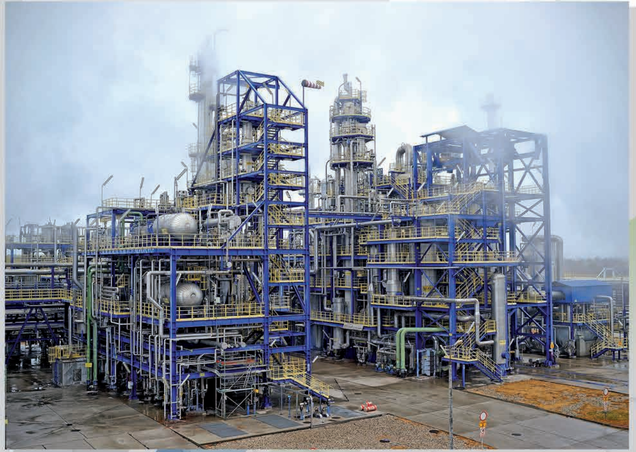
Construction of Melamine Manufacturing Plant III at Zakłady Azotowe "Puławy" S.A., Poland – project executed as General Contractor
