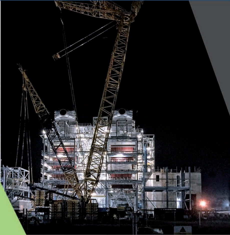
Erection of two boilers (26 MW e ) together with equipment and grates at waste incineration plant (capacity 275 000 t/year) in Beddington (South London), UK
